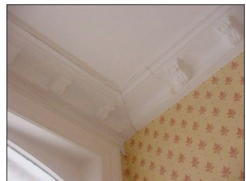
Hairline cracking in entrance hall
