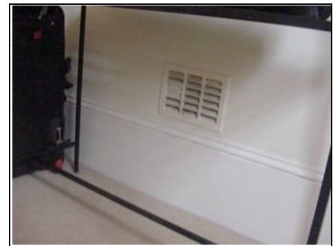
Vent to chimney rear left hand side
