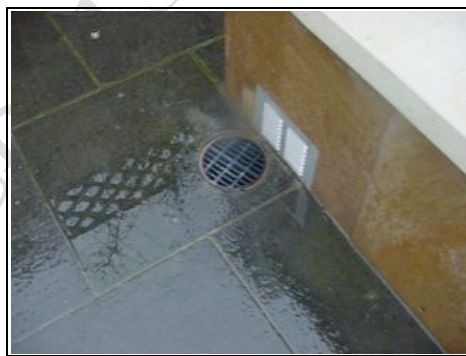
Airbrick acting as a gutter
