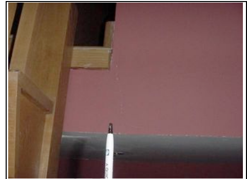
Hairline cracking on the stairway on top floor
