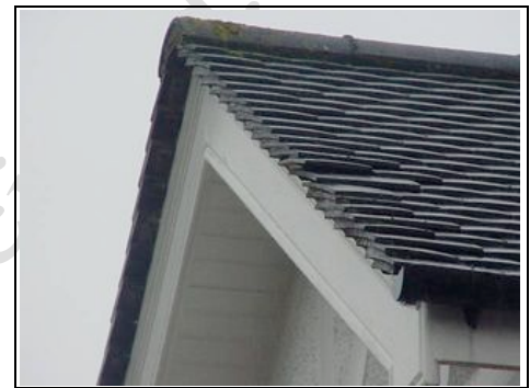
Tiles slightly displaced to the front
