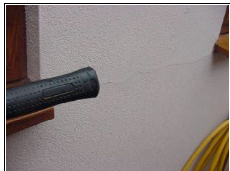
Cracking to the render
