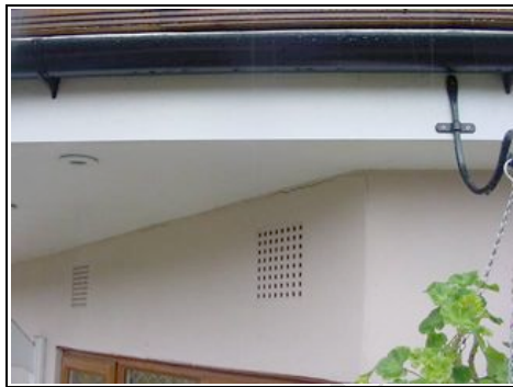
Crack at high level
