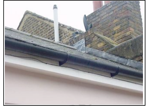
Soil and vent pipe
