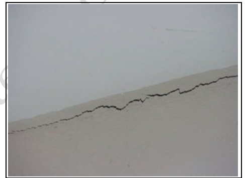
Close up of crack at high level
