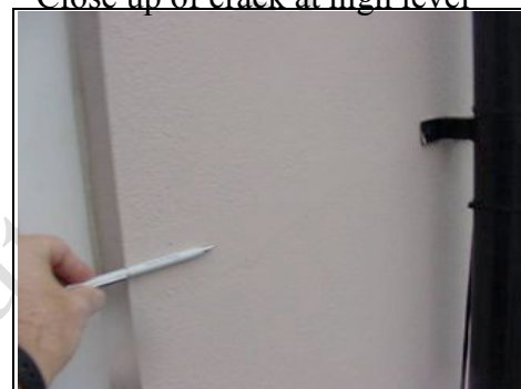
Old cracks that have been repaired previously
