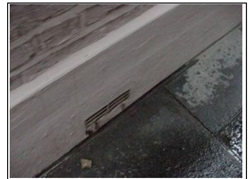
Airbrick acting as a gutter on the right hand side
