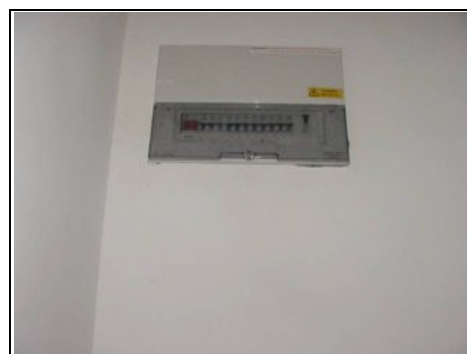
Fuse Board on first floor
