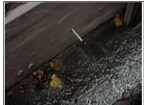
Damp proofing on right hand side
