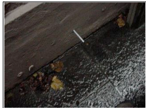
Damp proofing on right hand side
