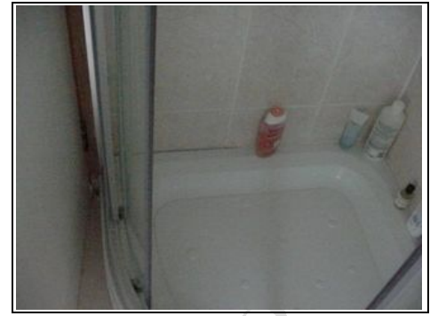
Deterioration to shower
