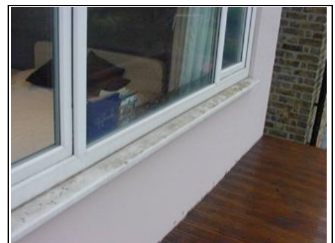
Wood decking covering the roof. Here we can see where the decking meets the main wall where there is no flashing
