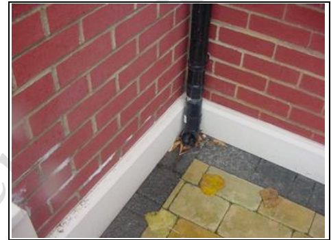
Plastic downpipe discharging onto the ground
