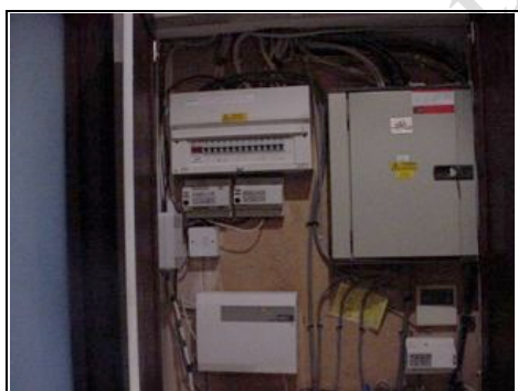
Circuit board on ground floor
