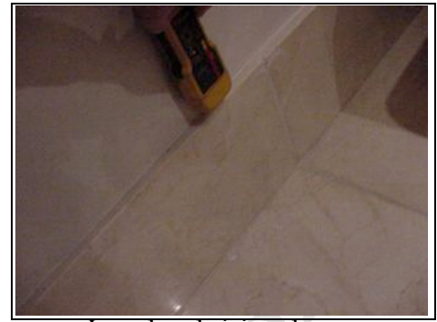
Low level rising damp
