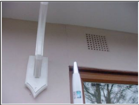
Crack in the render to the rear
