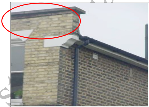
'Drip detail' on older property
