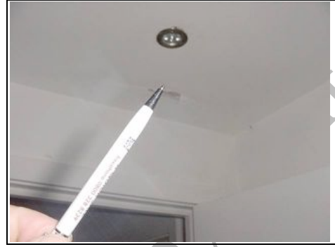
Dampness coming through the ceiling
