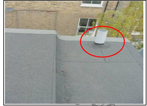
Flue from internal soil and vent pipe
