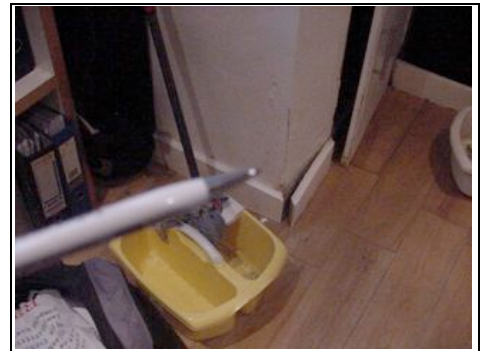
Dampness to adjoining Wall
