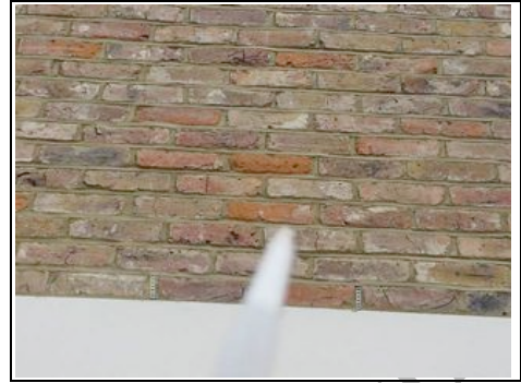
Cracking in brickwork
