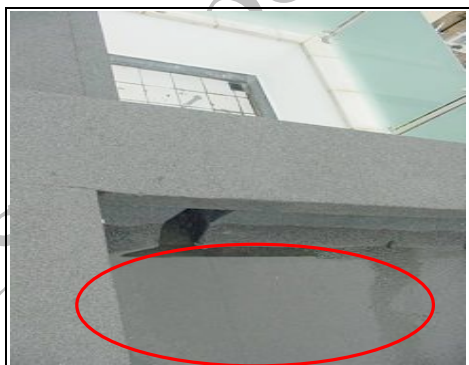
Ponding on roof
