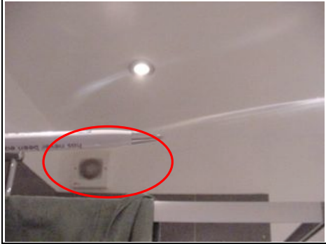
Extract fan is too small
