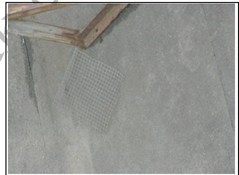
Mesh that used to cover downpipe outlets
