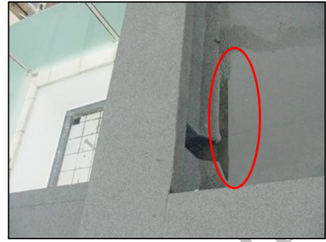
Water sits on the roof
