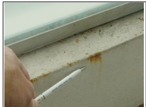
Balcony Internal bead being used externally
