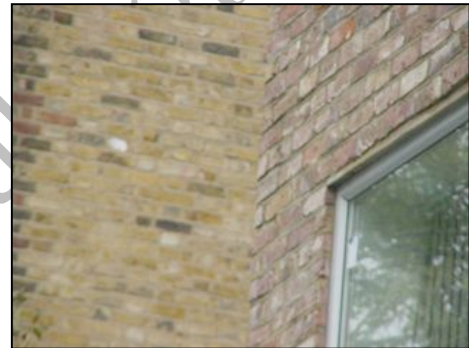
Window may be too far forward
