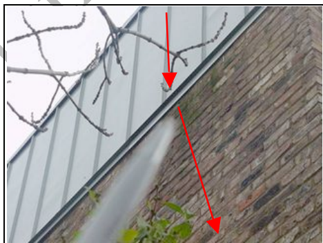
Water discharges onto the brickwork
