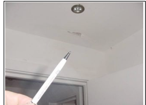
Dampness coming through the ceiling
