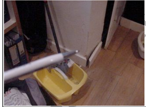
Adjoining wall affected by damp
