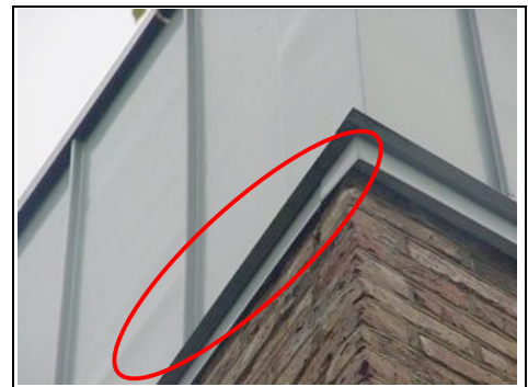
Front and side- poor drip detail- water discharges onto the brickwork
