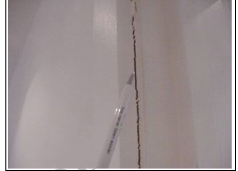
Door leading to balcony cracking visible
