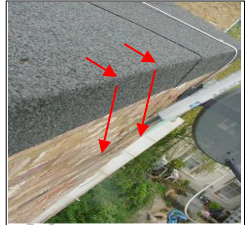
Rear of property – no drip detail Rainwater will discharge down the wall
