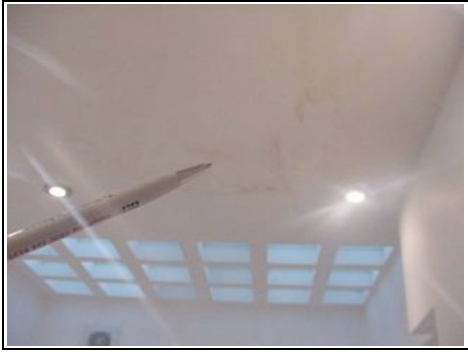
Staining to ceiling
