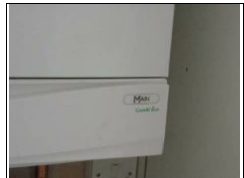
Wall mounted Main boiler
