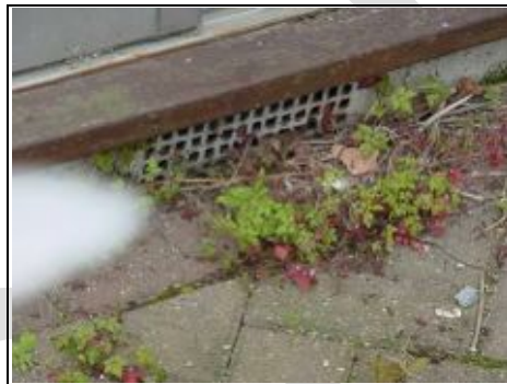
Air brick may be acting as a gutter
