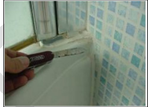
Shower is leaking
