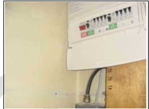
Electric fuse board
