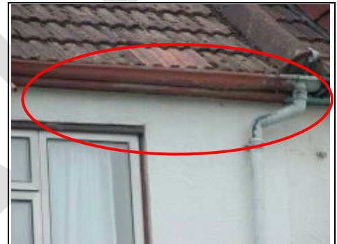
Gutters and downpipes need redecoration
