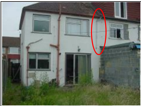
Downpipe discharging down the wall to the rear causing dampness
