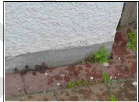
No DPC visible
