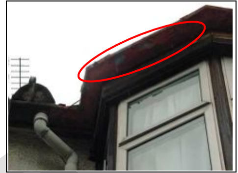
Gutters need re-decoration
