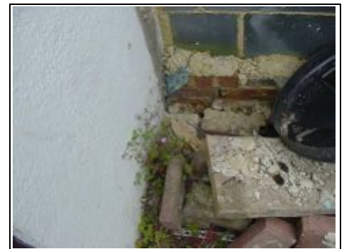
Where is the drain for the rainwater pipe to the rear?
