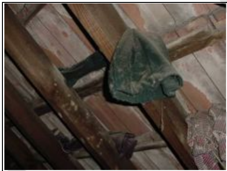
Rags filling gaps in roof
