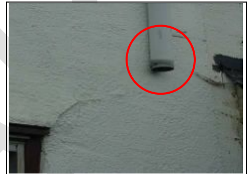
No outlet to join into at ground level
