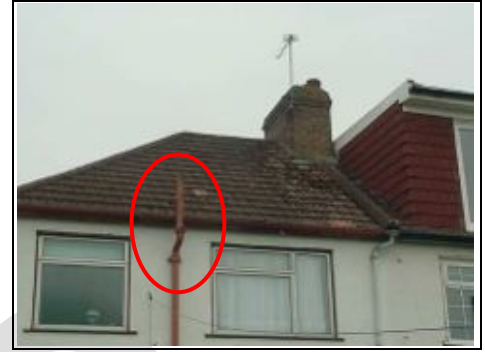
Soil and vent pipe
