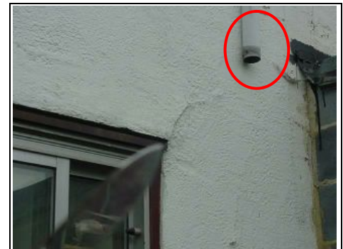
Down pipe with nowhere to discharge into
