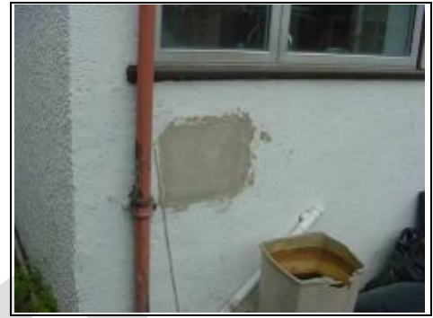
Render needs repairs and painting where the old boiler was removed
