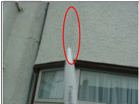
Hair line crack to the property
