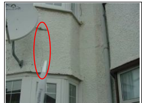
Hair line crack to the neighbouring property (left)
