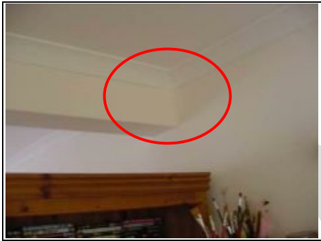
Wall removed without a pier support
