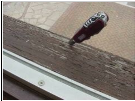
Timber is in poor condition
