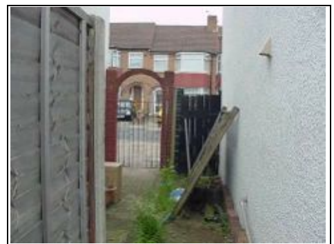
Fence has fallen down to right hand side
