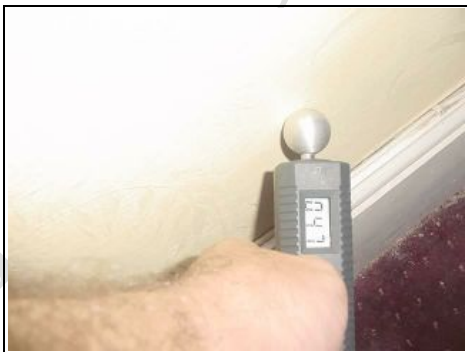
Damp reading is what we would expect to the front wall
