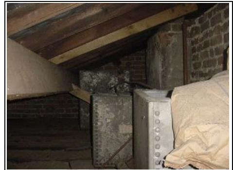
Water tanks need to be removed
