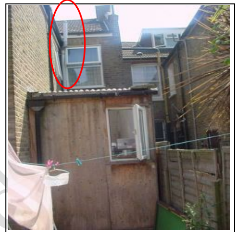
Soil and vent pipe
