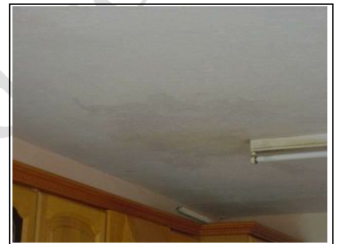
Ceiling damage in the kitchen
