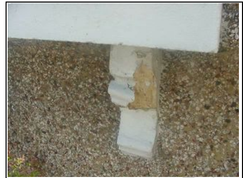
Damage to corbel
