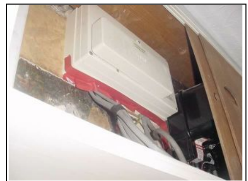
Electric fuse board
