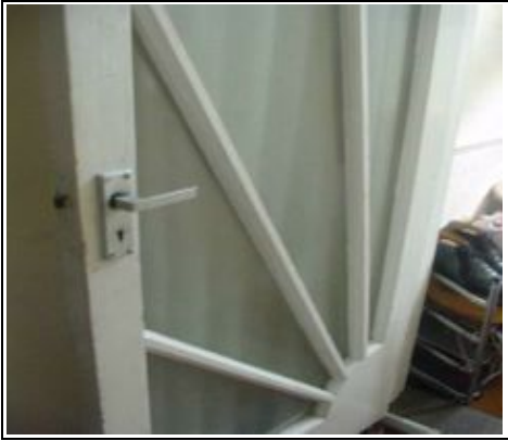
No safety glass in entrance door
