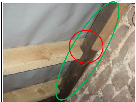
New timbers have been cut incorrectly (red circle) where they meet the wall plate (green oval)
