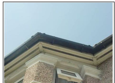
Vented fascias and soffits
