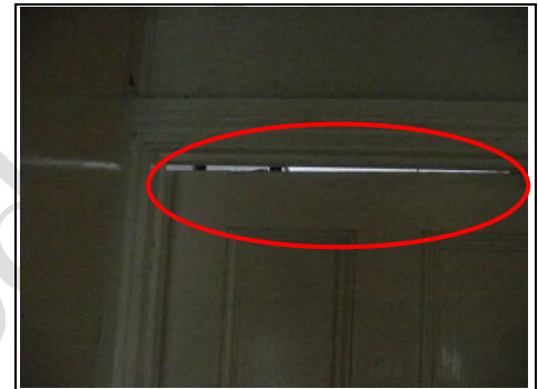
Gap showing movement above the front bedroom door
