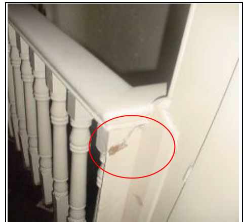
Damage to balustrade on landing needs repair
