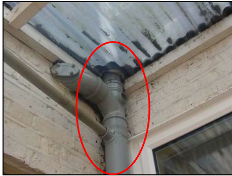
Soil and vent pipe in lean-to
