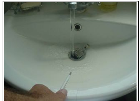
Sink is cracked
