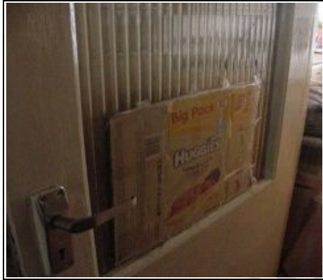
Crack in glazed door
