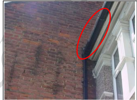
Overflowing gutter and downpipe
