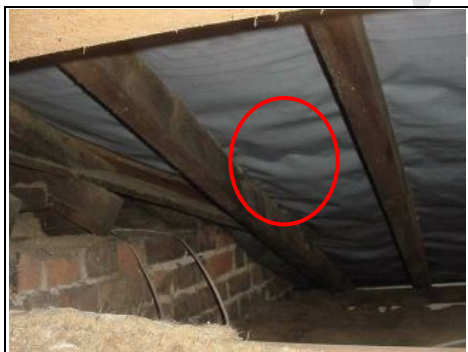
Dampness in roof may be condensation
