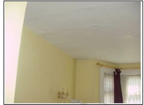
Paper is coming away from the ceiling in the lounge
