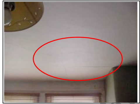
Cracking to front lounge ceiling
