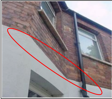
Incorrect detail where render meets brickwork allows the water to travel down the back of the render
