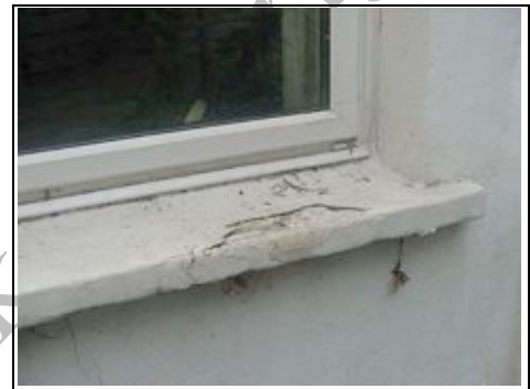
Window sills need repair
