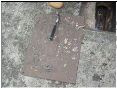
Rusting manhole cover
