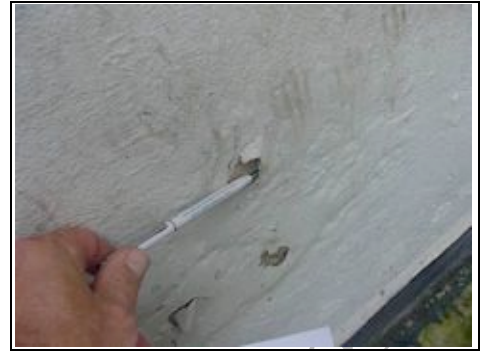
Blistering due to the use of plastic based paint
