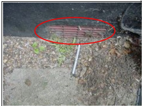
Air brick acting as a gutter
