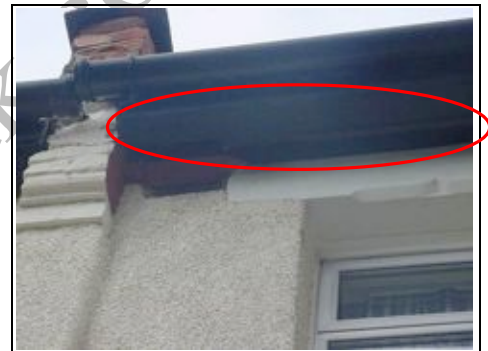
Timber fascias and soffits
