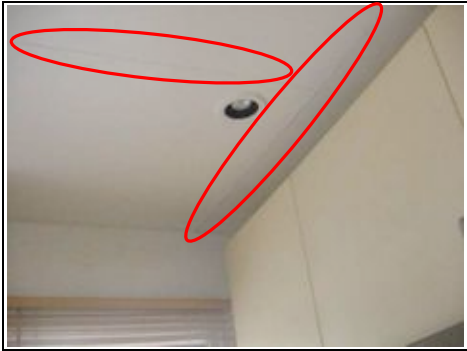
Cracking to the plasterboard in the kitchen
