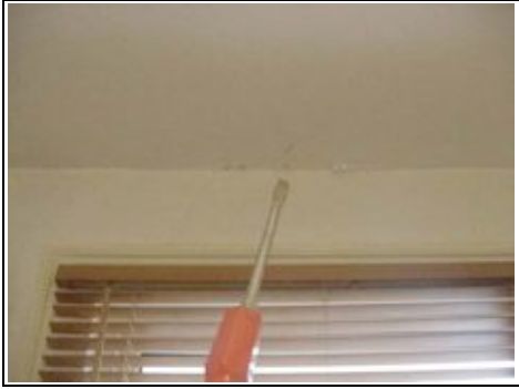
Peeling paint visible in bathroom caused by condensation
