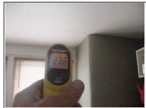
Surface temperature, 23.6 The difference in readings indicates cold bridging
