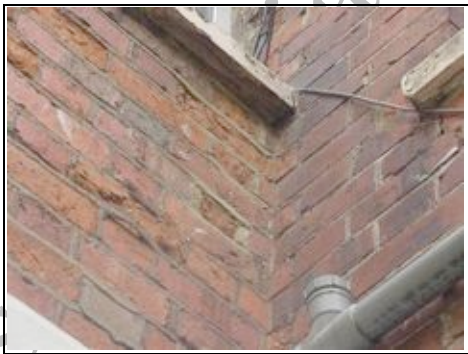
Spalling brick work
