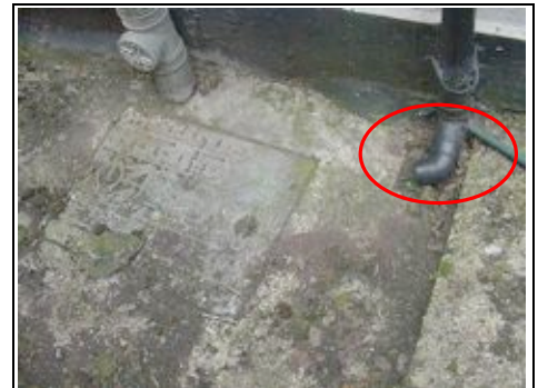
Downpipe discharging into partially blocked drain
