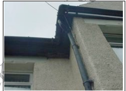
Plastic gutters and downpipe
