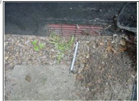
Air brick acting as a gutter
