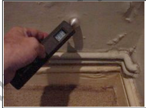
High damp readings
