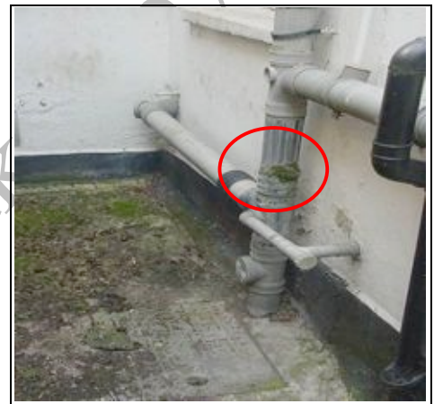
Soil and vent pipe is leaking
