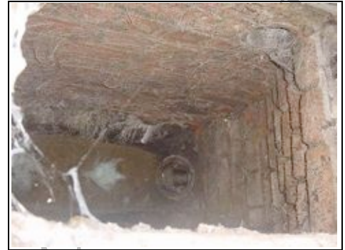
Roots in the front manhole
