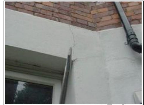
Cracking around window
