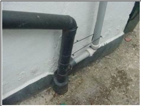
Cable ties holding plumbing together
