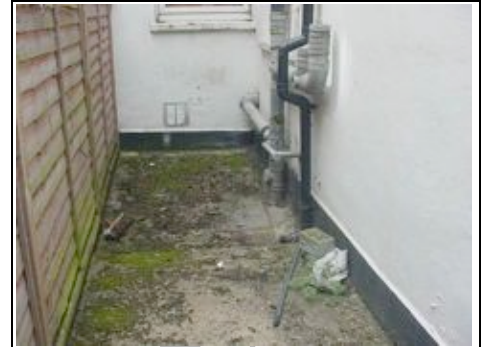
Soil and vent pipe
