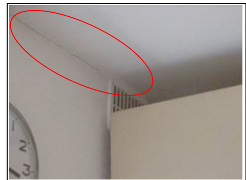
Cracking where walls meet the ceiling
