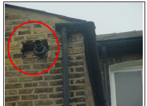
Flue from a boiler
