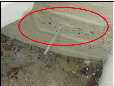
Airbrick to the front needs unblocking to allow airflow under the suspended timber floor
