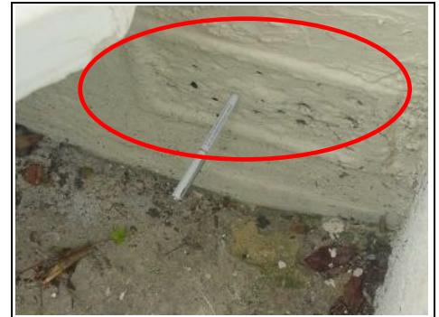
Airbrick to the front needs unblocking to allow airflow under the suspended timber floor
