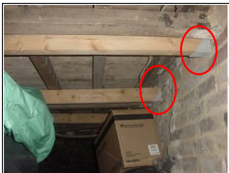
New timber beams supporting the floor with joist hangers on the right hand side
