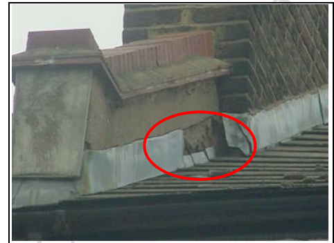
Lead flashing has come away
