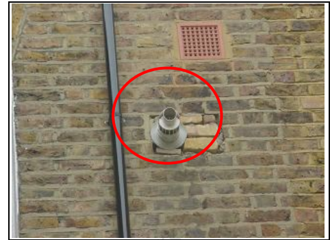
Flues have not been blocked in properly
