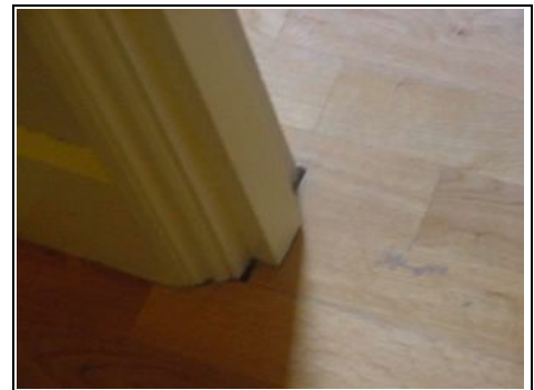
Laminate flooring over the suspended timber floor. This does not have the best quality finish
