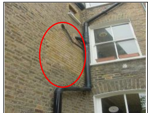
Flemish bond brickwork with an area of patched brickwork
