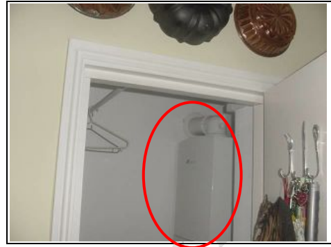
Worcester boiler in the service cupboard/utility area
