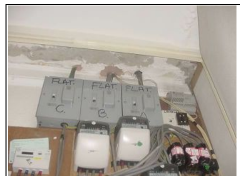
Main electric fuse board cupboard
