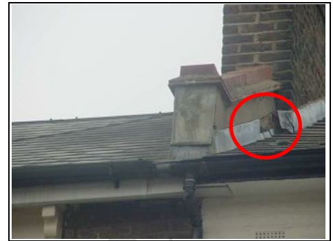
Parapet wall- lead flashing has come away (front left)
