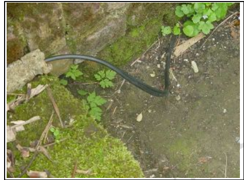
Exposed cable in garden
