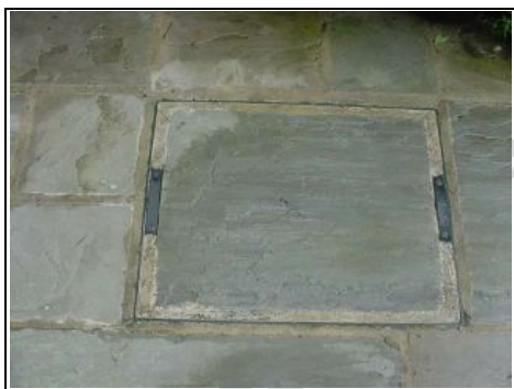
Drain to the rear We did not lift this
