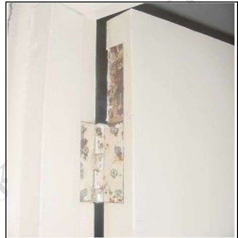
Hinge has been moved on the door
