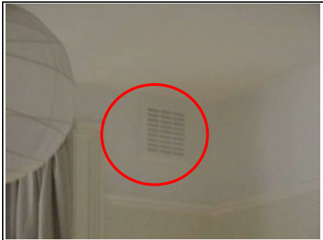
High level air vent
