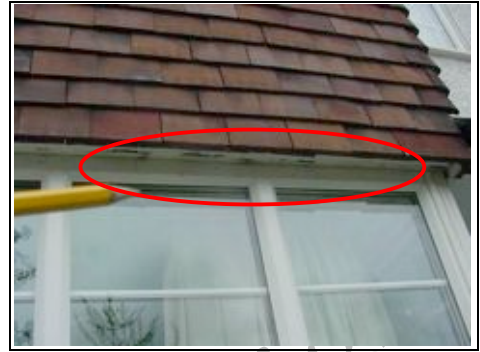
Windows need sealant
