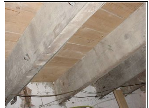
The ceiling of the cellar is also the ground floor suspended floor.
