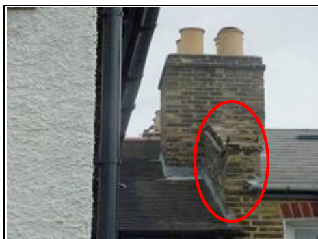
Rear left parapet wall is difficult to see
