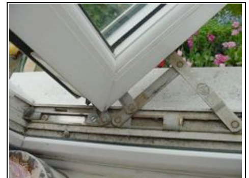
Rusting to the window hinges
