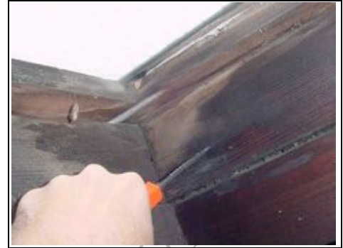
Roof window, dampness is coming in
