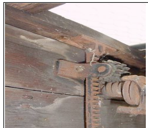
Mechanism for opening the window has rusted
