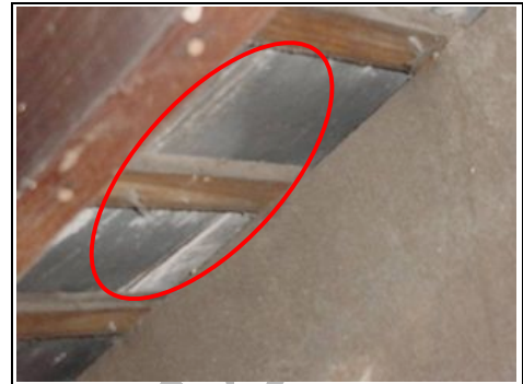
Slates are visible where the protective underlayer has deteriorated (see the next section)
