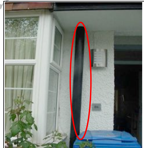
Plastic soil and vent pipe for the en suite shower room
