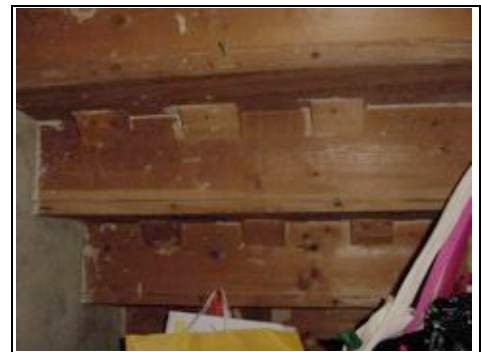
Stairs are not lined
