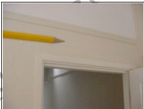
Hairline cracking above and to the side of the door to the master bedroom
