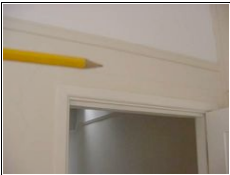
Hairline cracking above and to the side of the door in the master bedroom
