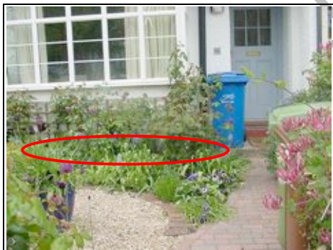
High ground level, the airbricks have been covered over
