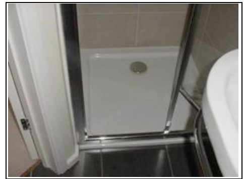
Shallow shower tray, there can be problems with these overflowing
