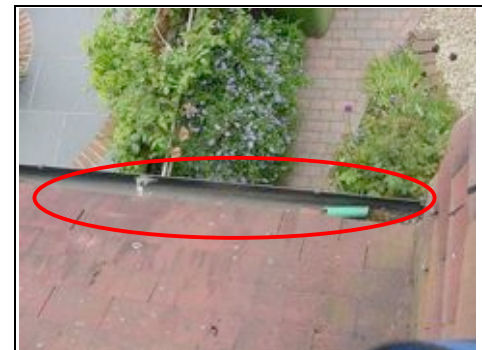
Clear the gutter. We are always mystified by what ends up in the gutters
