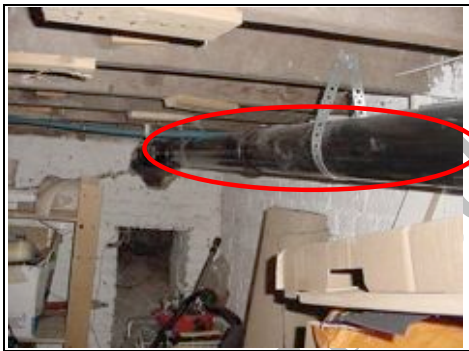
Soil and vent pipe visible from en suite shower room in cellar
