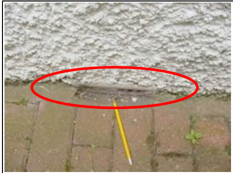
Air brick is too low (rear left)
