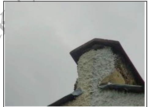
Rear right parapet wall
