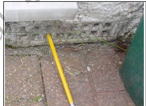
Air brick to the rear is too low
