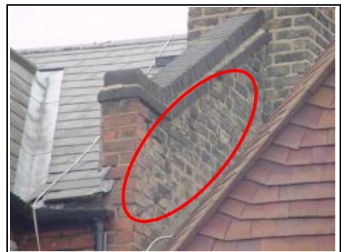
Left parapet wall needs re-pointing
