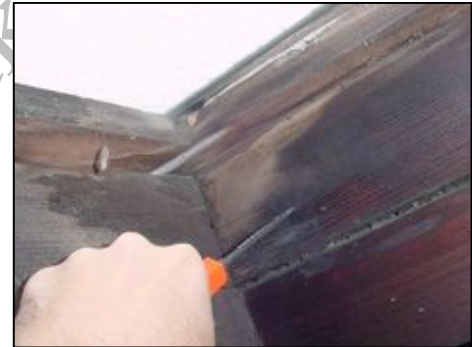
Roof window is allowing dampness in
