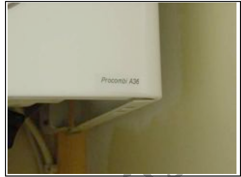
Procombi A36 boiler
