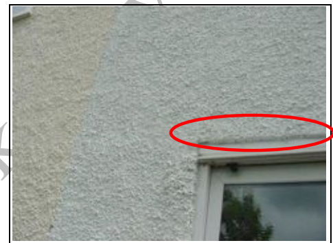
No window drip
