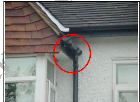
Plastic gutters and downpipes
