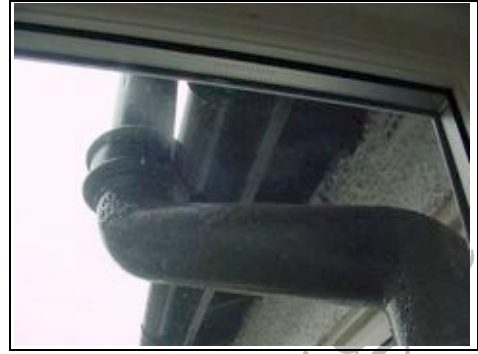
Cast iron soil and vent pipe
