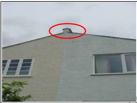
Rear right parapet wall
