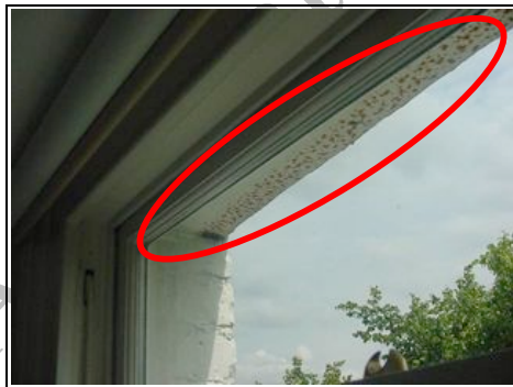
Rusting to lintel
