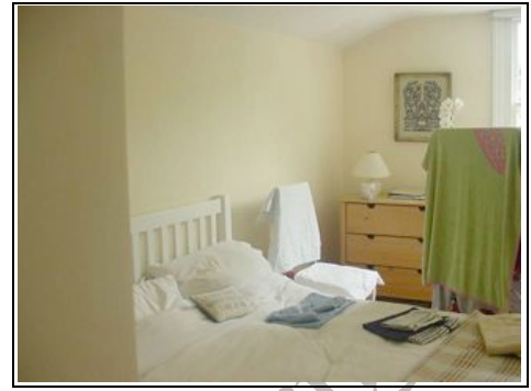
Mold is formed partly within the roof
