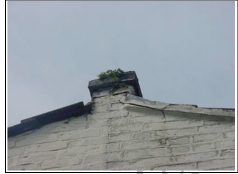
Growth of vegetation to rear parapet
