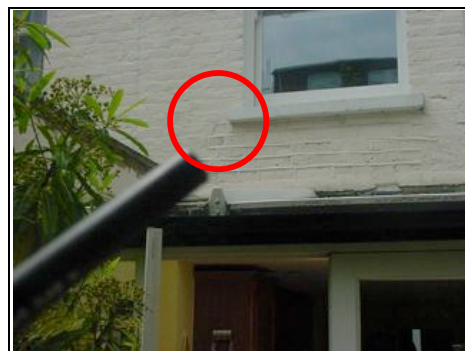
Crack in brickwork
