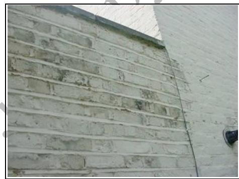
Rear low level parapet wall in need of redecoration
