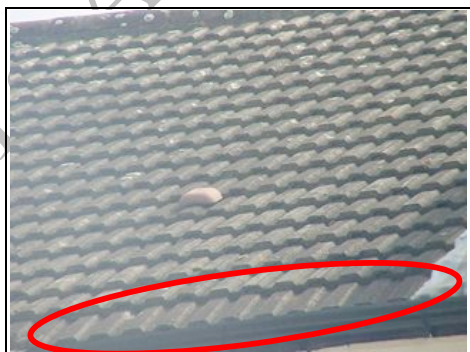
Concrete roof tiles – no tilting fillet
