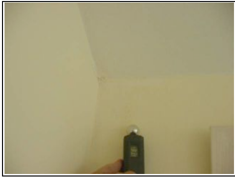
Damp areas which we believe relate to cold bridging
