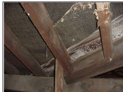
Dampness coming from rear valley gutter
