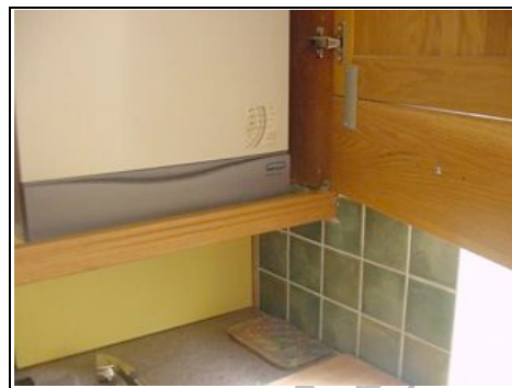
Older style Potterton boiler
