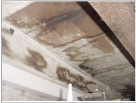
Dampness noted in cellar to the suspended timber floor/ joist and floorboards
