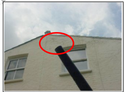
Cracking to rear of property at high level
