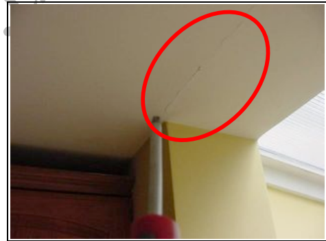
Plasterboard crack to ceiling
