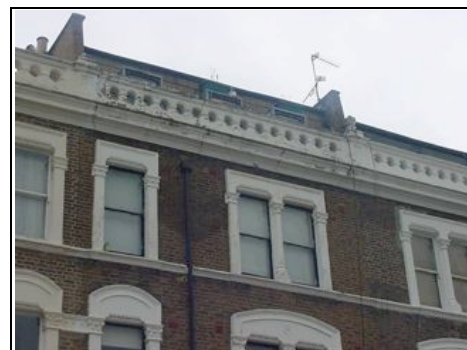
Classic Victorian Sliding sash windows where they have managed to put in one pane of glass
