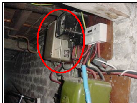
Older part of electrics
