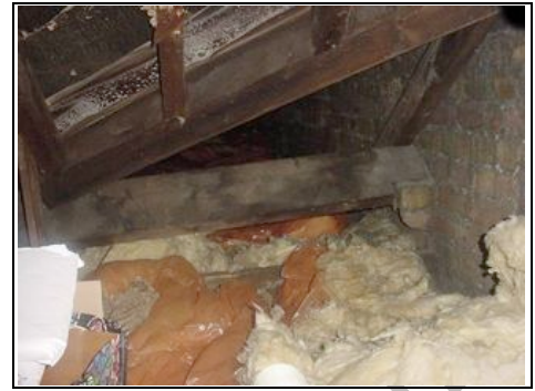
Looking towards rear roof Discolouration on joists which we think is from condensation
