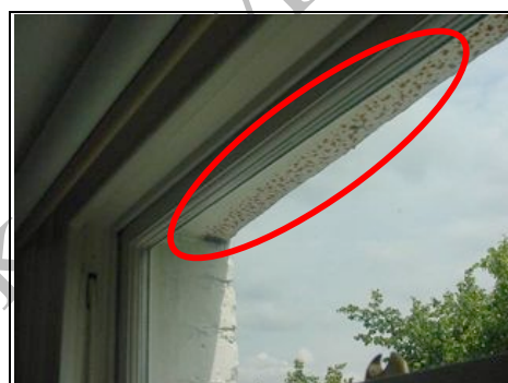
Rusting metal lintels
