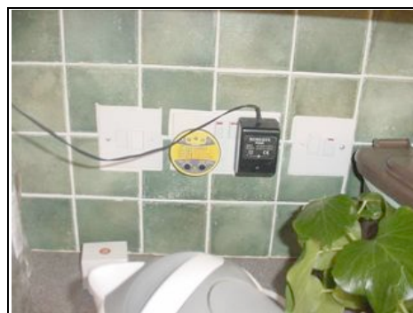
Earth test failed
