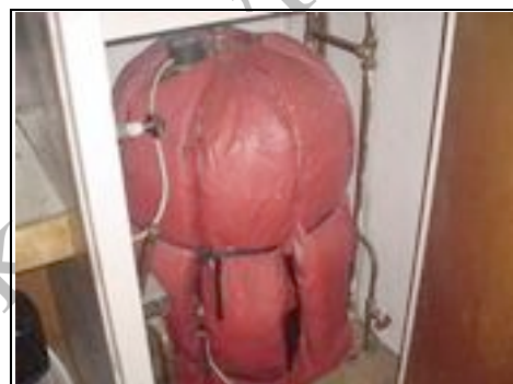
Older style cylinder with loose insulation jacket
