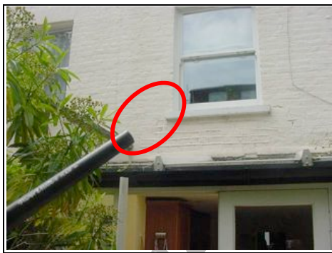
Cracking to rear of property at low level
