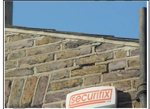
Ad hoc repointing required to rear of property
