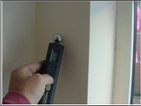
Dampness in kitchen
