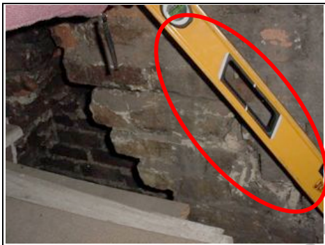
Crack to chimney
