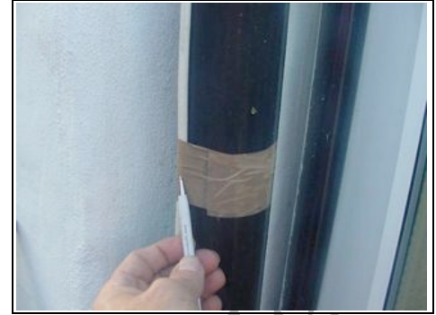
Electrics taped to wall
