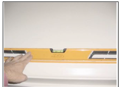
Top of door out of alignment
