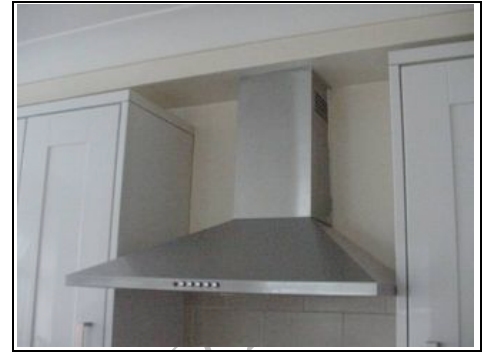
Filter in kitchen, not an extract
