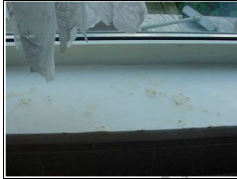
Flaking of paint to window sill in kitchen
