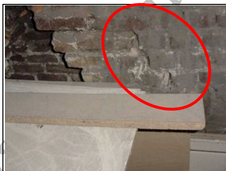
Crack in chimney
