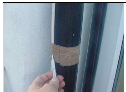
Electrics taped to wall
