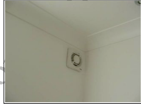
Small extract in bathroom needs to be bigger
