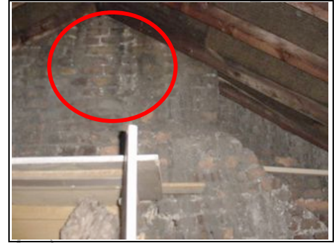
Dampness coming in via front left chimney
