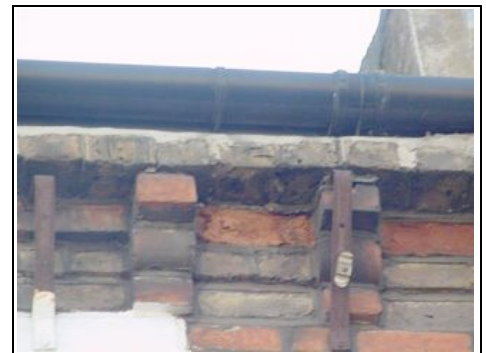
Spalling to soft red brick
