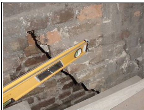
Close up of crack
