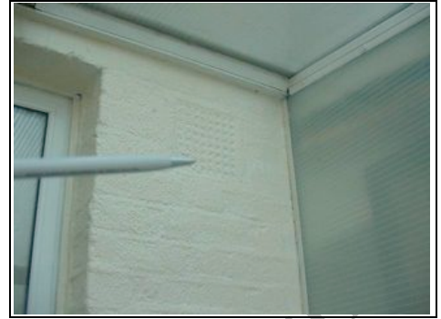
Blocked high level vent
