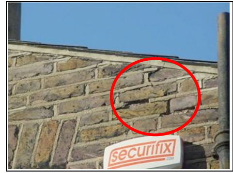
Cement mortar coming away
