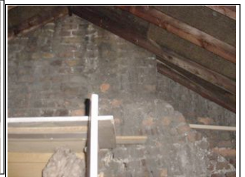
Dampness coming in via front left chimney
