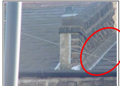
Crack in next doors side which will allow dampness into your property
