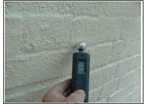
Dampness to utility room/outside cupboard area
