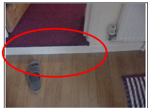
Step in kitchen where we believe vent should go
