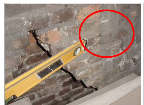
Close up of crack
