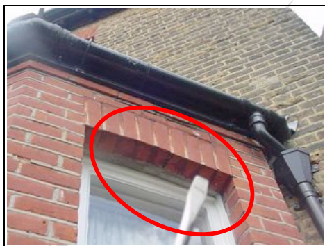
Soldier course above window has moved
