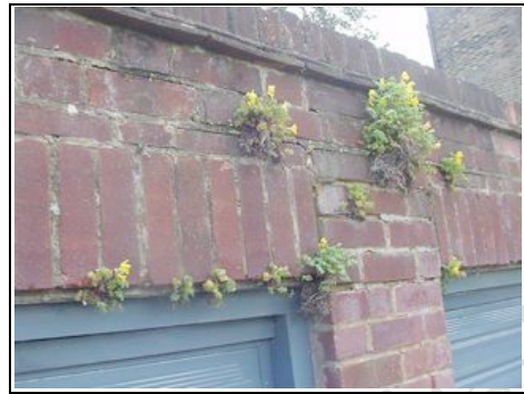
Plants growing from garage wall
