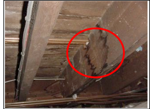
Leak from above or condensation from the pipes
