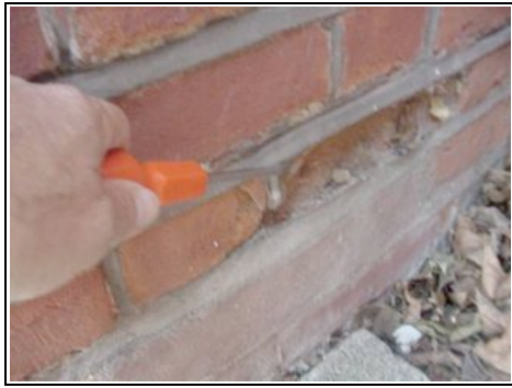
Spalling of brickwork caused by cement mortar
