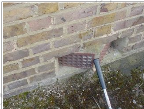
Unusual double vent which leads us to believe that the floor joists have been laid in different directions
