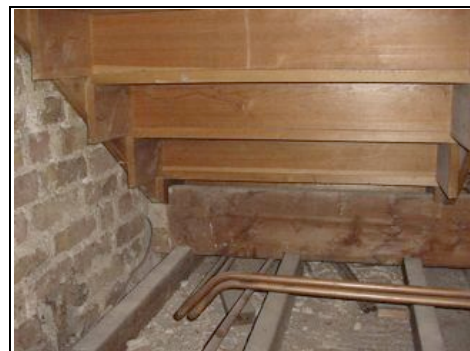
Unprotected staircase from first floor to second floor seen within roof above kitchen.
