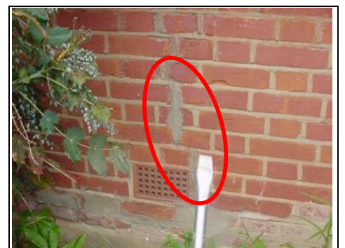
Cracking to rear bay window
