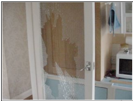
How the door initially cracked
