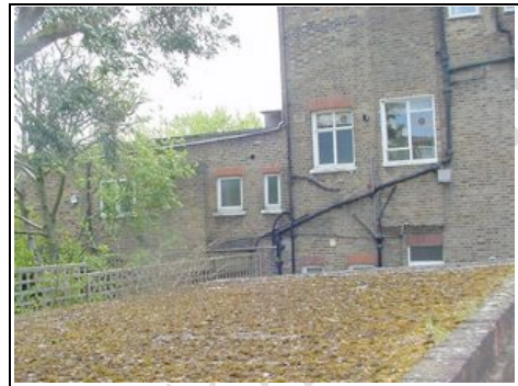
Deterioration to all the asbestos garage roofs
