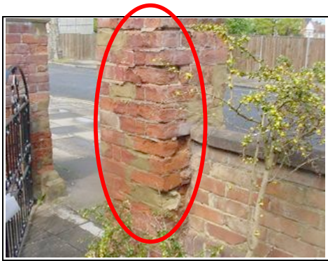
Boundary wall in poor condition, repaired with cement
