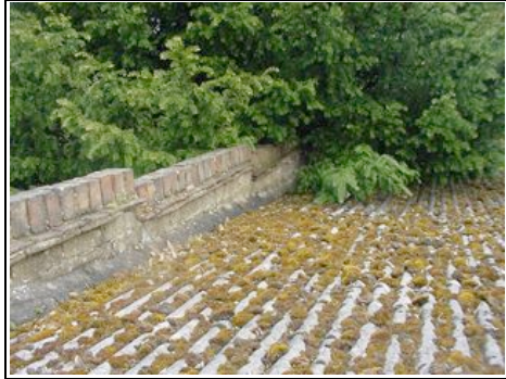
Deterioration to your asbestos garage roof
