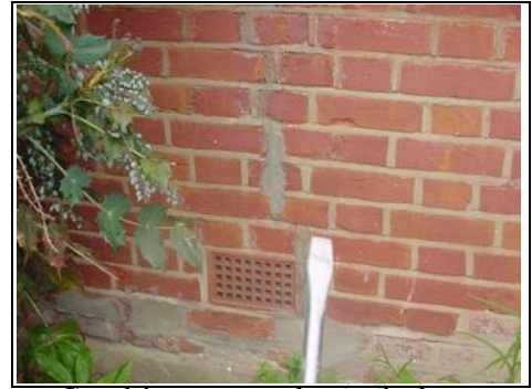
Cracking to rear bay window
