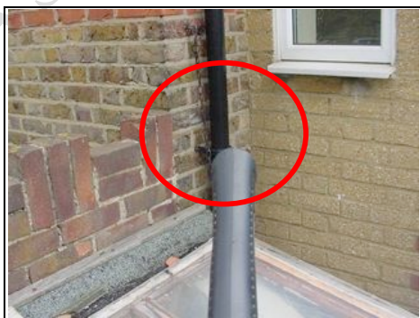
Crack between original building and rear bay
