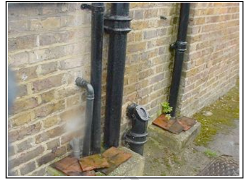
Soil and vent pipe
