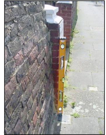
Level shows how far out boundary wall is
