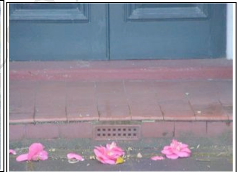
Airbrick acting as gutter at front door
