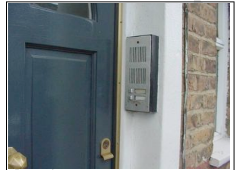
Door entry system to other flats
