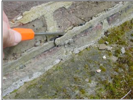
Cement mortar coming away
