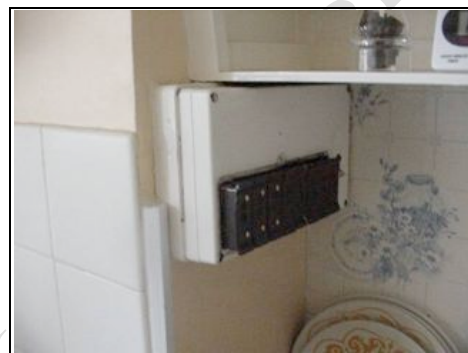
Dated fuse board
