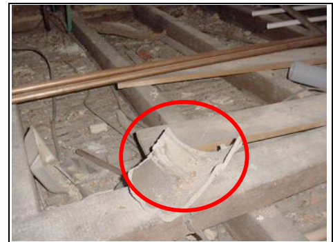
Asbestos in kitchen roof
