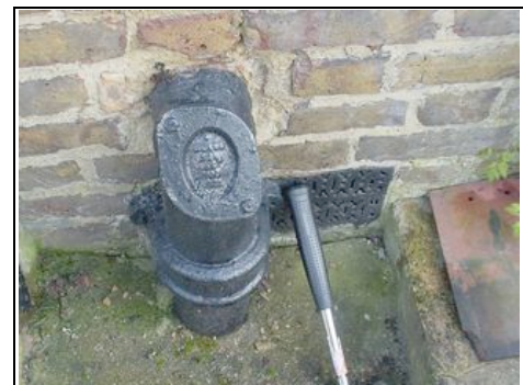
Vent to right hand side wall
