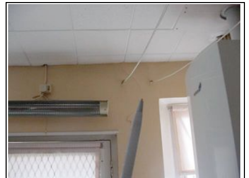
Crack in kitchen wall
