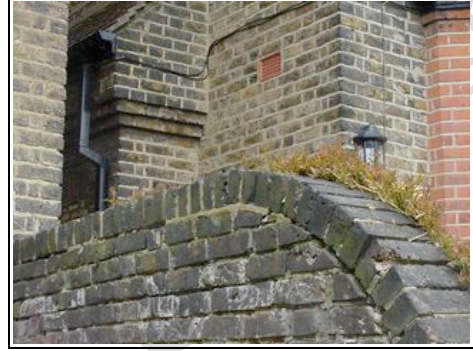
Plant life growing on wall and needs repointing
