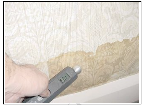
High damp meter readings on right hand side of property
