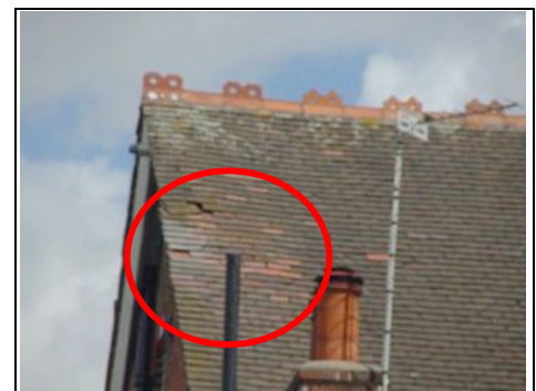
Perimeter tiles that are missing are often caught by the wind and lifted
