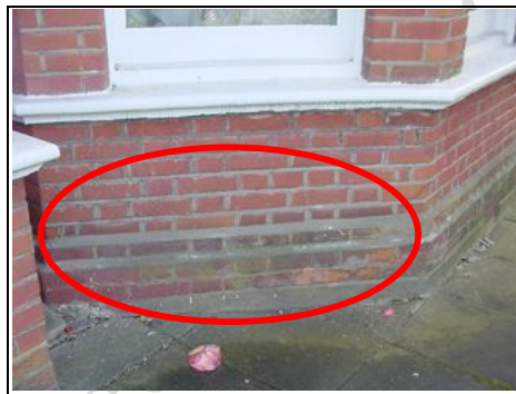
DPC to older part of property. Thickening of brickwork indicates slate dpc originally
