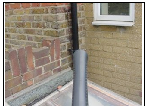
Crack between original building and rear bay
