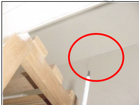
Crack in airing cupboard next to bathroom
