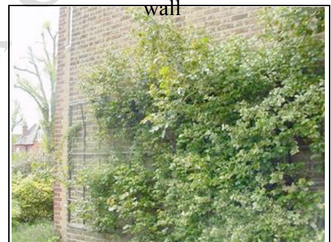
Plant growing on wall which needs maintaining
