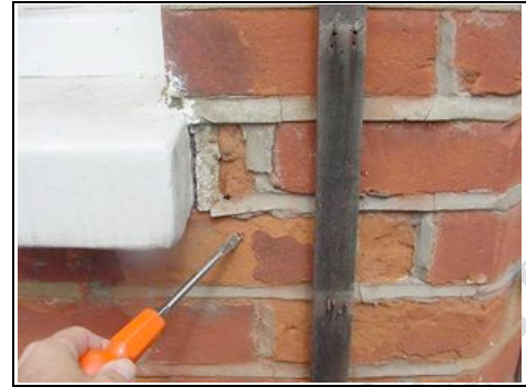
Spalling to brickwork caused by cement mortar
