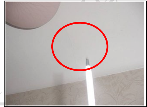
Hairline crack to lath and plaster in hallway
