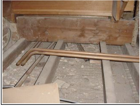
Unsupported copper pipes in roof above kitchen
