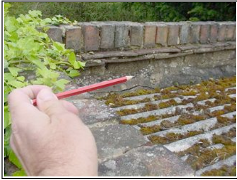
Cracking to the cement flashing surrounding asbestos
