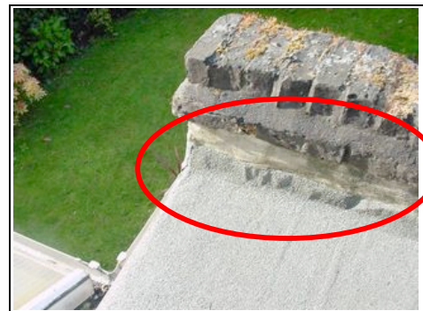
Felt flashing is also not particularly good and may be attributing to dampness getting in
