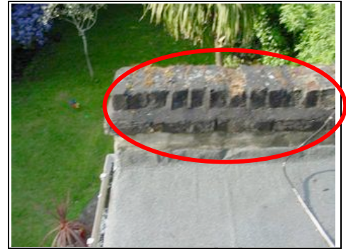
Parapet wall which is causing problems to flat below
