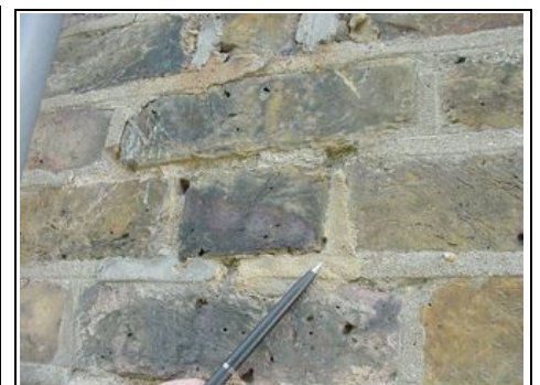
A mixture of cement and mortars including the pen pointing to the more modern very hard cement mortar
