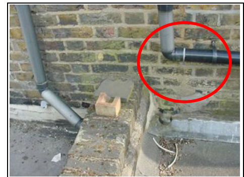
Sharp bend on the rear rainwater downpipe which we tend to find
