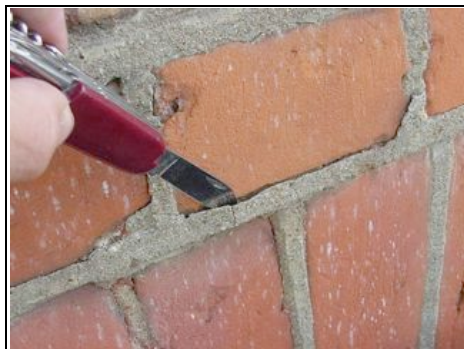
Cement mortar coming away
