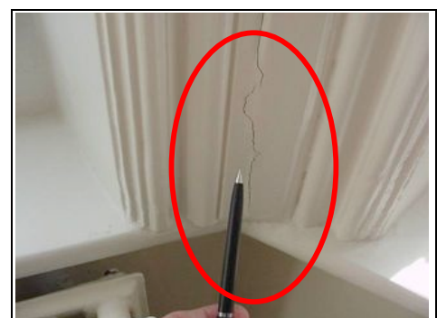
Cracking to front bay
