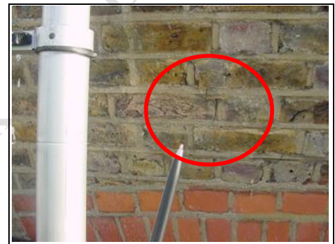
Cracking to rear
