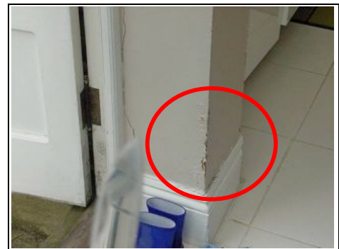
Rising damp to ground floor apartment
