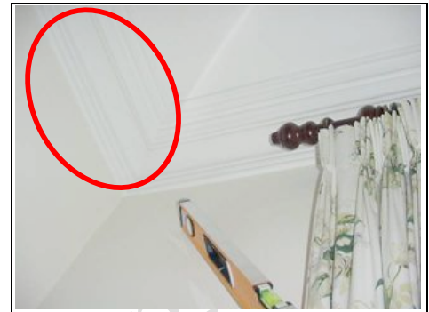
Cracking to rear right bedroom
