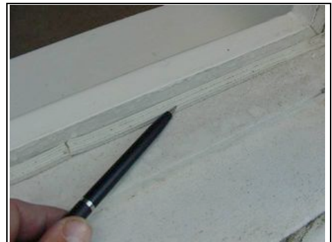
Only seal we found on windows 17 for sealing draughts
