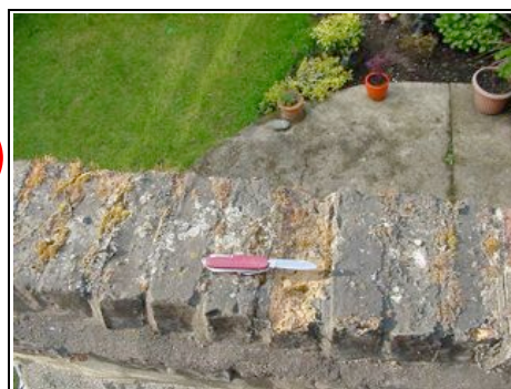
Deterioration to parapet wall
