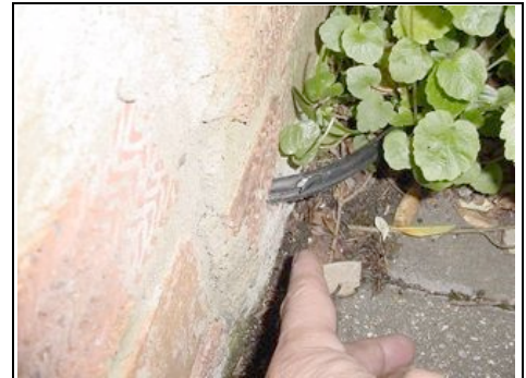
Cable outside coming through wall
