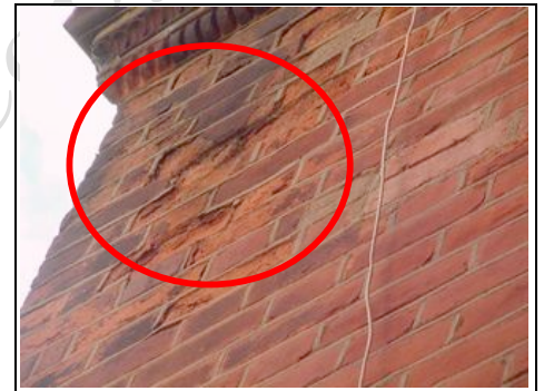
Spalling brickwork at high level
