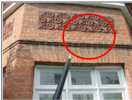
Cracking above bay window
