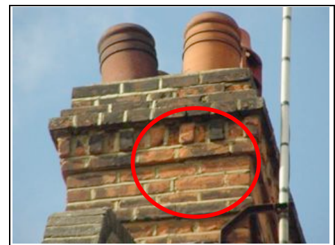
Spalling brickwork to chimney one
