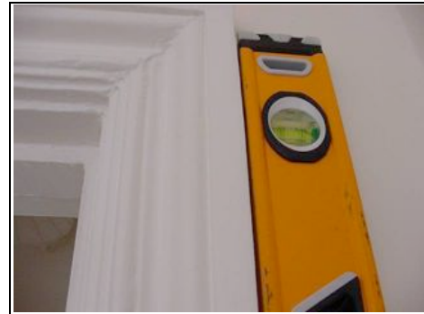
Rear bedroom door slightly out
