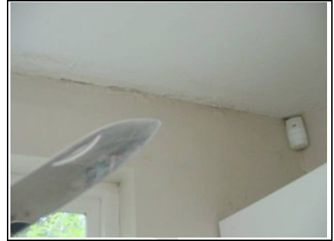
Dampness coming in from parapet wall
