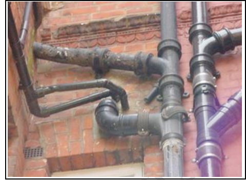
Soil and vent pipe
