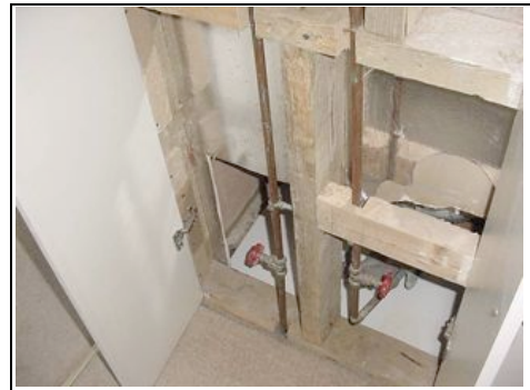
Cupboard to back of bath within hallway
