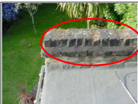
Parapet wall which is allowing water into flat below
