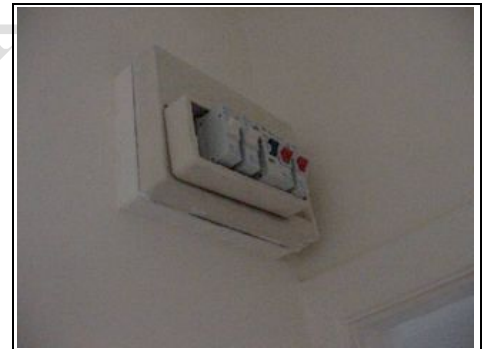
Fuse Board in apartment
