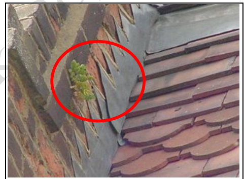
Plant growing from parapet wall on left hand side
