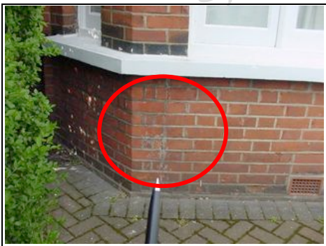
Cracking to front bay
