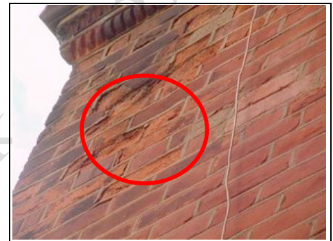
Spalling brickwork at high level
