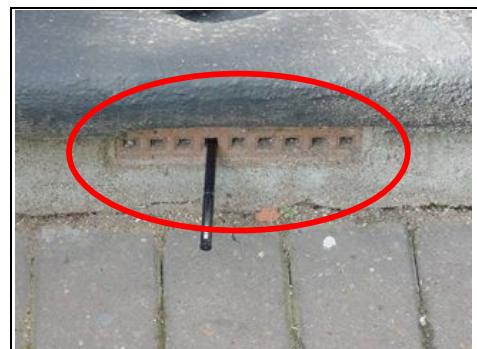
Air brick too low
