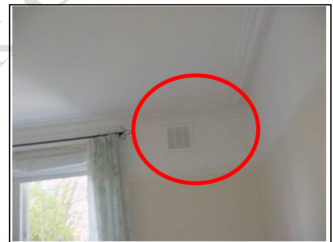
High level air vent
