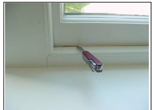
Windows not fitting very well
