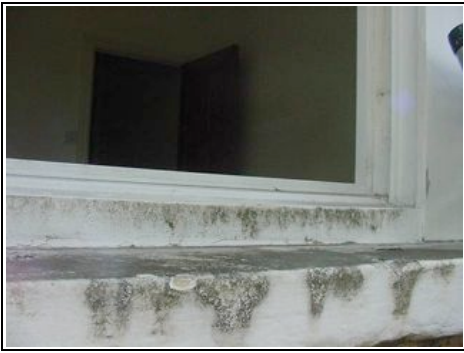
Window sills need painting
