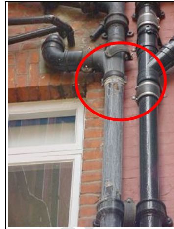
Sewerage pipe leaking
